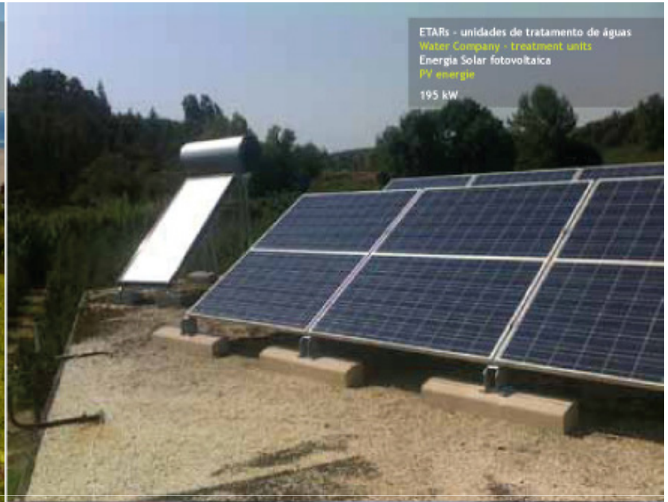
Hotel turismo senior Hotel senior tourism Fotovoltaico e AQS Photovoltaic and water heating 24 kW
